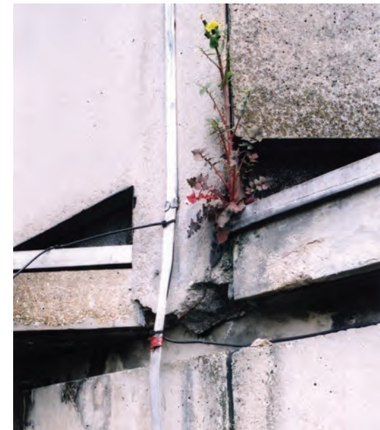
Precast concrete panels on a ziggurat block showing their age.
