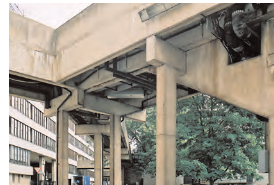
Main service runs are located under the walkways.
