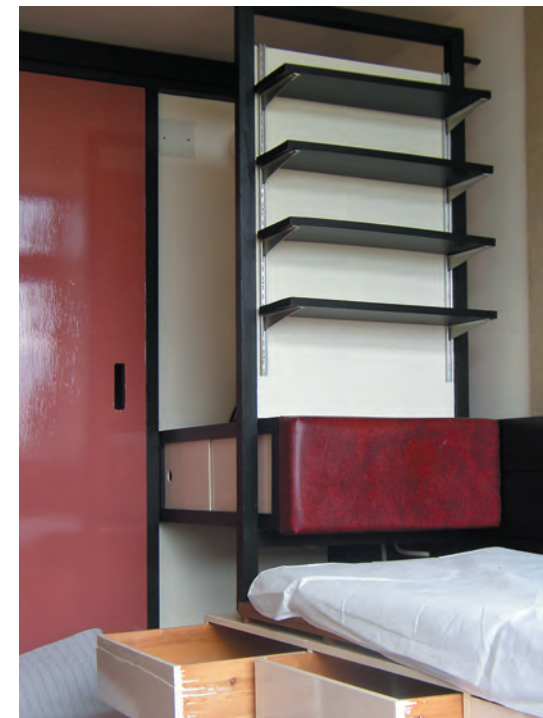
Some of the original study fittings are worn and in need of refurbishment.
