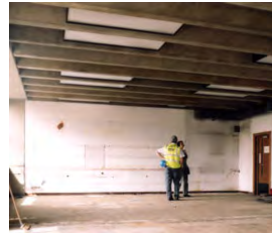
The Academic Wall is constantly being refitted for changing academic needs. The column-free spaces can be used in many different ways. This space has a ceiling formed by Lasdun's unpainted precast floor slabs, and his purpose-made lights. (2006)
