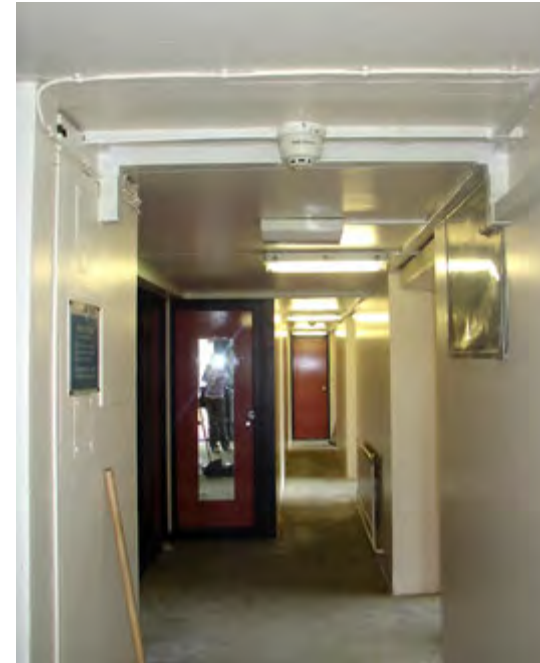
The corridors in the ziggurats are tightly dimensioned and have become cluttered with surface-mounted lights and services. (2006)
