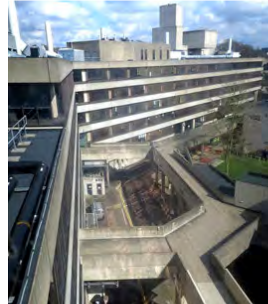
The roof and raised walkway viewed from the lecture room on the roof of Sciences, looking towards Chemistry and Arts I. (2018)
