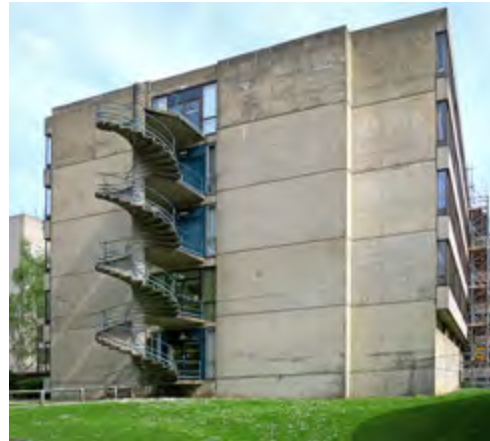
Other ends of building and service towers left 'open' for extensions (Arts spur [3] shown). (2018)
