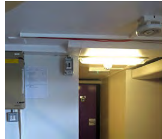
Surface-mounted services in the ziggurat corridors [105, 106]. (2018)
