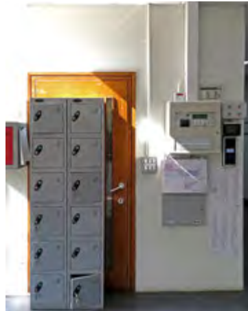
Numerous adhoc alterations for partitions, services, fixtures and finishes. (2018)
