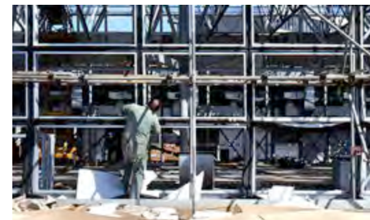
Assembly of the SCVA superstructure: neoprene gaskets being placed between the subframes on which the cladding panels are mounted. (photo June 1977)
