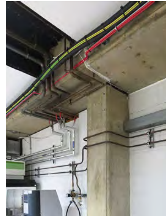
Adhoc accumulation of services in the Academic Wall, no longer accommodated by the service ducts provided in the original construction. (2018)
