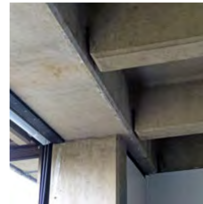
Primary structure of precast concrete (Ladsun zones [3, 4, 6], shown) or in-situ concrete (F&M zones [3, 5]). (2018)
