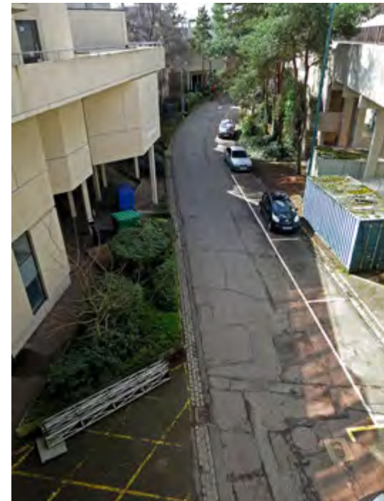
The north side of Norfolk Terrace [106]. The precast concrete panels of the ziggurat have been painted coated . (2018)
