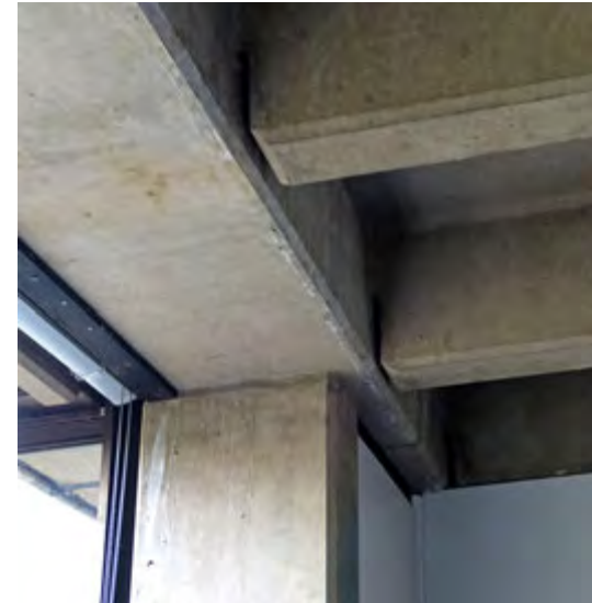
The precast structure of the Lasdun zones with U-shaped vertical columns enclosing vertical ducts, edge beams between columns with recesses for blinds, and floor slabs of wide planks with T-shaped downstand ribs. The ribs align with the window mullions. (2018)
