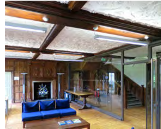
The central hall in Earlham Hall, divided by a glazed screen to create a fire escape route from the stairs. (2018)
