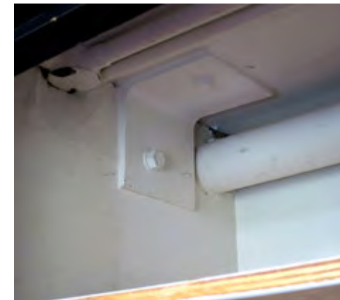
New brackets have been fitted to meet regulations (introduced after the original construction) preventing the progressive collapse of prefabricated buildings. They are unobtrusively located in cupboards, etc. (2018)
