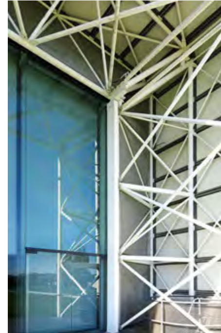
Between the end wall glazing and the external skin, grey panels are fixed between the triangulated structural members; they are poorly sealed and have poor insulation. (2018)
