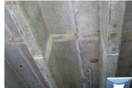
Underside of a Lasdun precast floor with traces of change – there is no need to obliterate traces which do not impair functionality and provide evidence of change over time. (2018)
