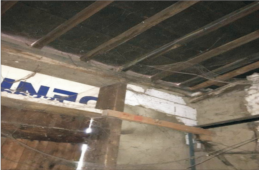
PHOTOGRAPH 11: Cobwebs around door frame Building B9
