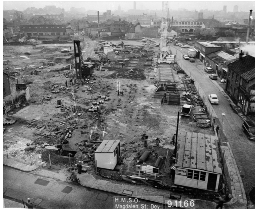
Figure 4.12 Anglia Square under construction in November 1966. Photograph taken from the original Odeon Cinema on Botolph Street, looking southwest Source: Reg Walker
