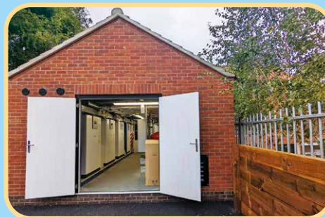
The new plant room
