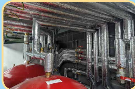
Part of the innovative heating system
