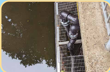
The heat source water pump
