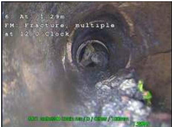
Photo: 39_39_275_A.jpg, 00:00:20 1.29m, Fracture, multiple at 12 O'Clock
