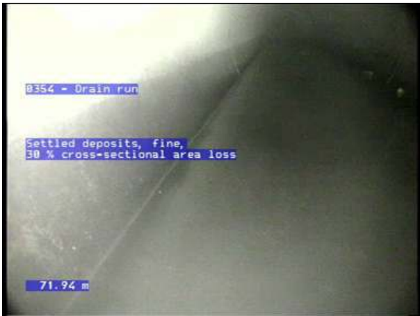
Photo: 30_30_217_A.jpg, 00:16:24 71.67m, Settled deposits, fine, 30 % cross-sectional area loss
