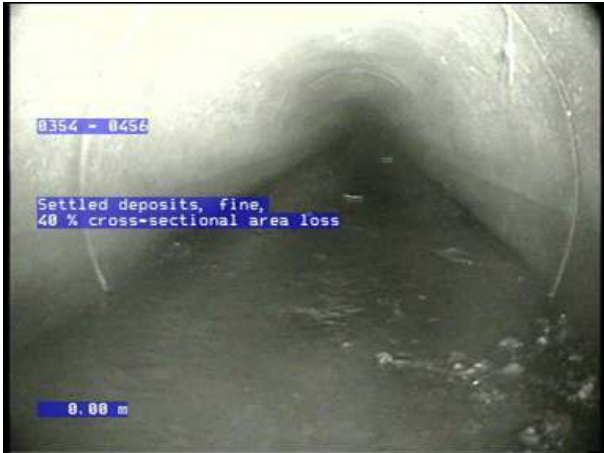
Photo: 29_29_204_A.jpg, 00:00:05 0m, Settled deposits, fine, 40 % cross-sectional area loss
