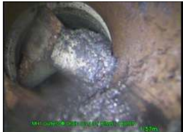
Photo: 39_39_276_A.jpg, 00:00:32 1.59m, Other obstacles, other at 12 O'Clock 70 % cross-sectional area loss debris / rubble
