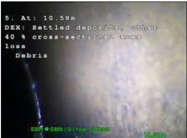
Photo: 6_6_26_A.jpg, 00:02:11 10.58m, Settled deposits, other 40 % cross-sectional area loss Debris
