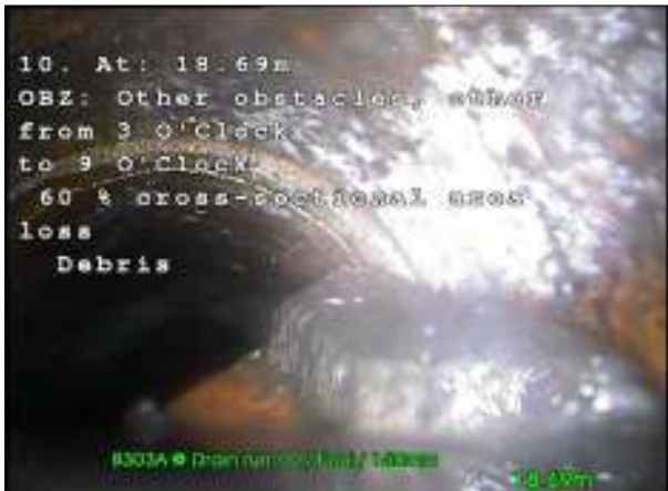
Photo: 21_21_153_A.jpg, 00:02:04 18.69m, Other obstacles, other from 3 O'Clock to 9 O'Clock 60 % cross-sectional area loss Debris
