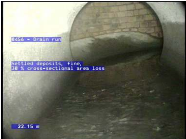
Photo: 28_28_197_A.jpg, 00:06:20 22.15m, Settled deposits, fine, 30 % cross-sectional area loss
