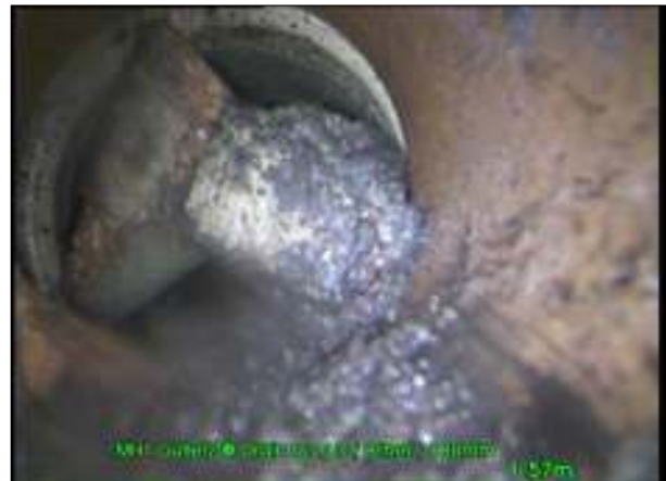
Photo: 39_39_276_A.jpg, 00:00:32 1.59m, Other obstacles, other at 12 O'Clock 70 % cross-sectional area loss debris / rubble
