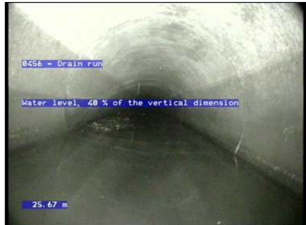
Photo: 28_28_200_A.jpg, 00:07:28 25.67m, Settled deposits, fine, 30 % cross-sectional area loss
