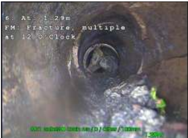
Photo: 39_39_275_A.jpg, 00:00:20 1.29m, Fracture, multiple at 12 O'Clock
