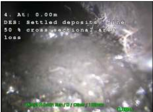
Photo: 42_42_301_A.jpg, 00:00:05 0m, Settled deposits, fine 50 % cross-sectional area loss
