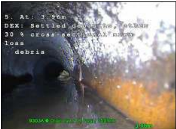
Photo: 22_22_157_A.jpg, 00:00:29 3.96m, Settled deposits, other 30 % cross-sectional area loss debris
