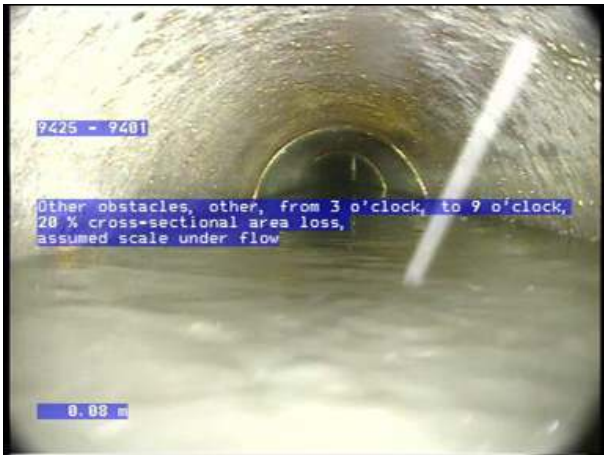
Photo: 36_36_254_A.jpg, 00:00:46 0.08m, Other obstacles, other, from 3 o'clock, to 9 o'clock, 20 % cross-sectional area loss, assumed scale under flow
