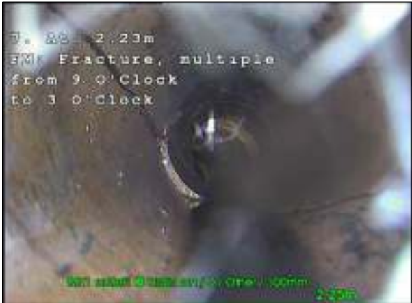
Photo: 38_38_263_A.jpg, 00:00:49 2.23m, Fracture, multiple from 9 O'Clock to 3 O'Clock
