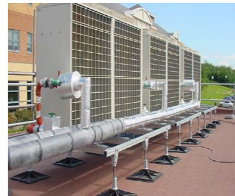
Rooftop AHUs for apartments and duplexes. NB they are to be concealed and not on show like this.
