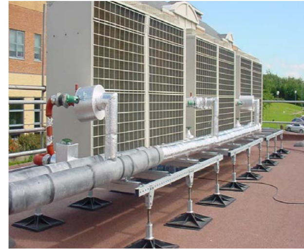
Rooftop AHUs for apartments and duplexes
