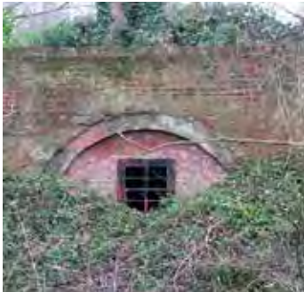
◀ A brick tunnel under Whitlingham Lane apparently through which chalk was taken along a railway to be loaded onto wherries. Evelyn Simak - geograph.org.uk
