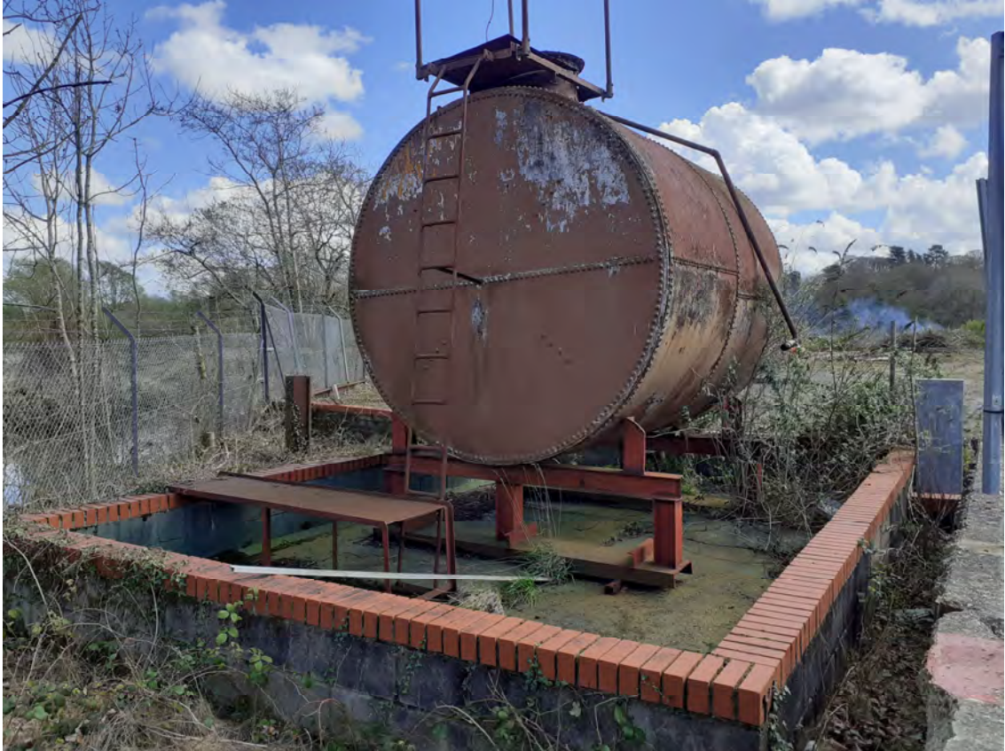
Photograph 28: 10000 litre bunded fuel tank close to northern boundary
