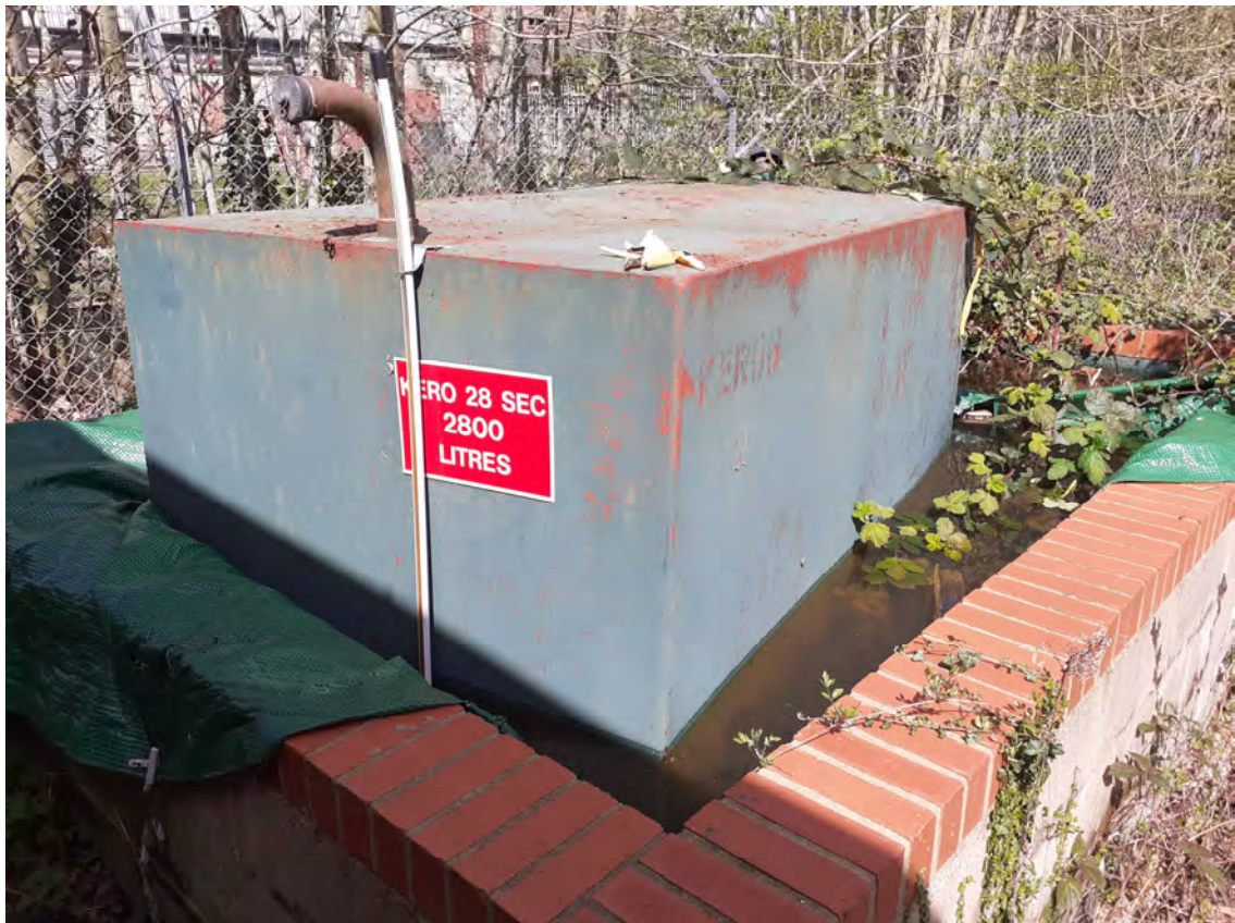
Photograph 21: Heating oil tank with bund full of water.
