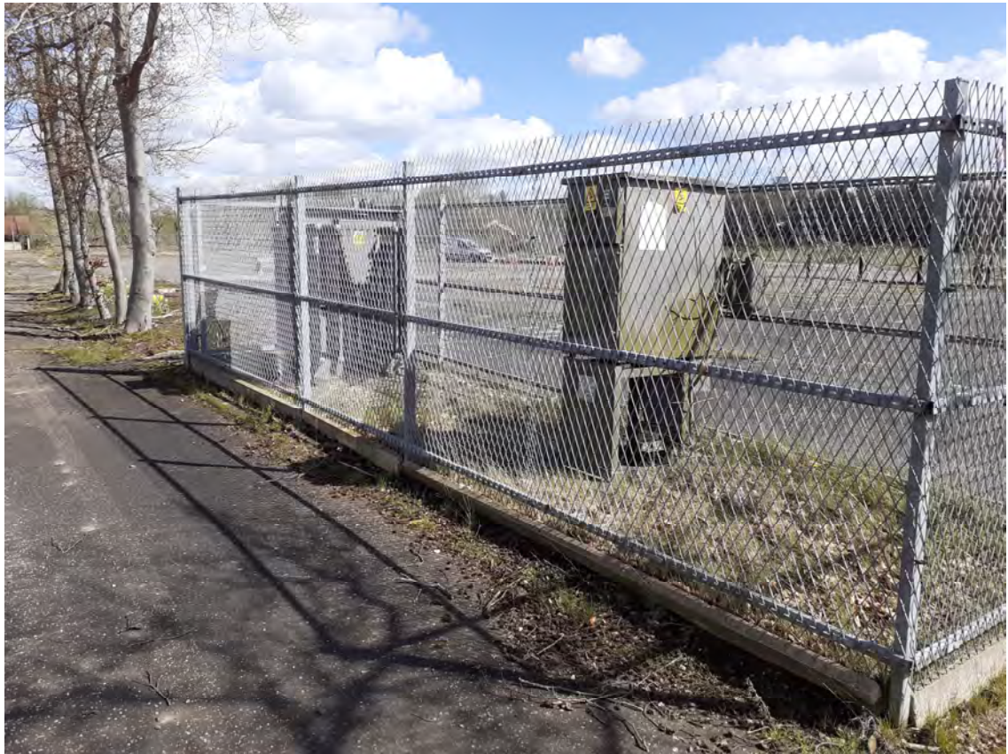
Photograph 24 : Substation to the west of the northerly office building
