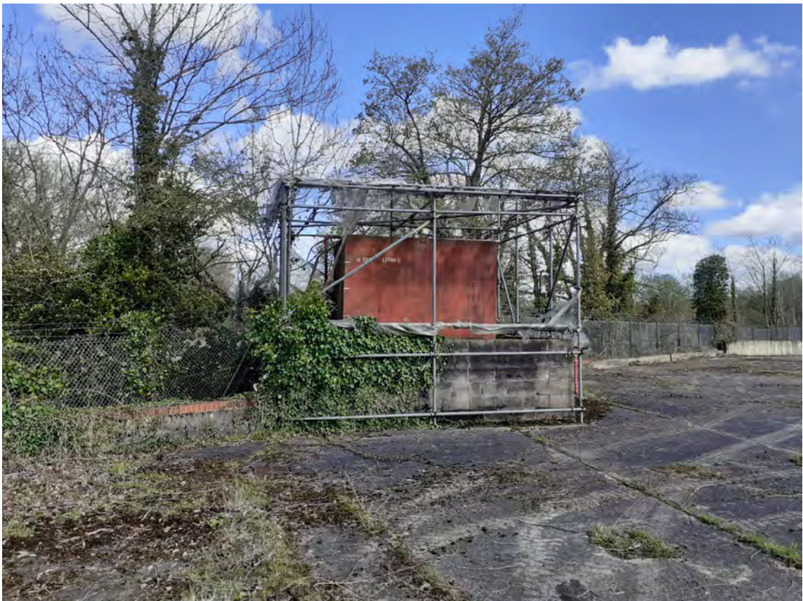
Photograph 27: 9000 litre bunded fuel tank
