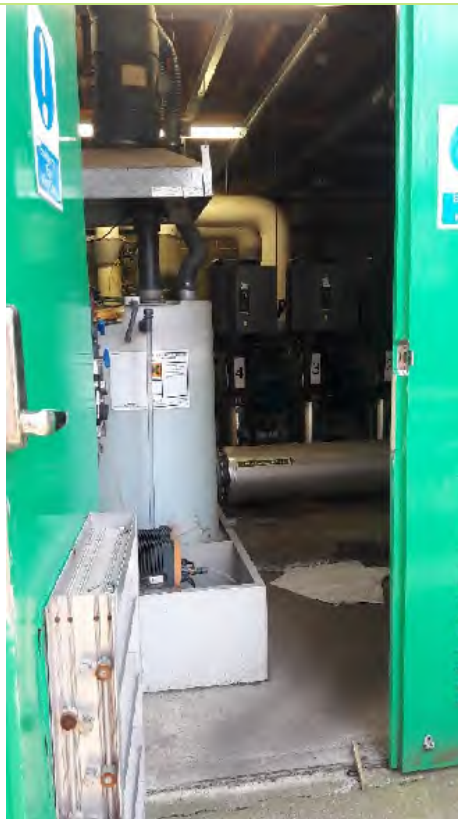
Plate 20: Internal part of the water treatment plant
