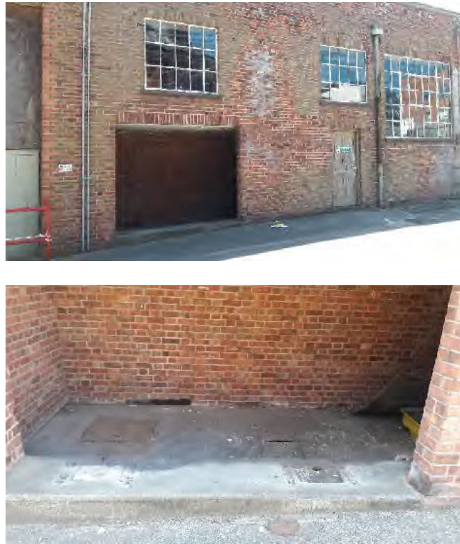
Plate 3: Building 207 in the northwest of the site. Evidence of former pumps, vent pipes and possible below ground tanks
