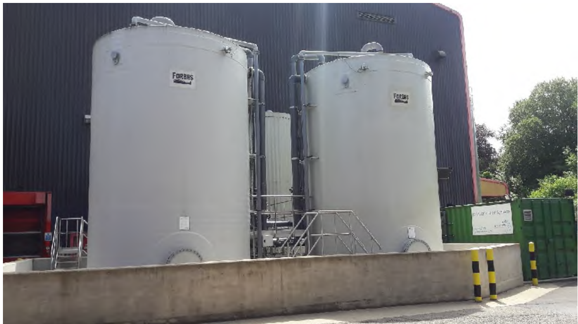
Plate 16: pH balancing plant to the west of building 254
