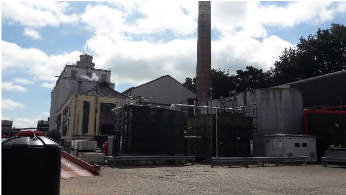
Plate 13: View of the sprinkler pump house (#256) with the boiler house and chimney behind. Tanks are for fire water storage (silver) and part of the water treatment system (green). BH 'F' and associated air stripping plant also located in this area.
