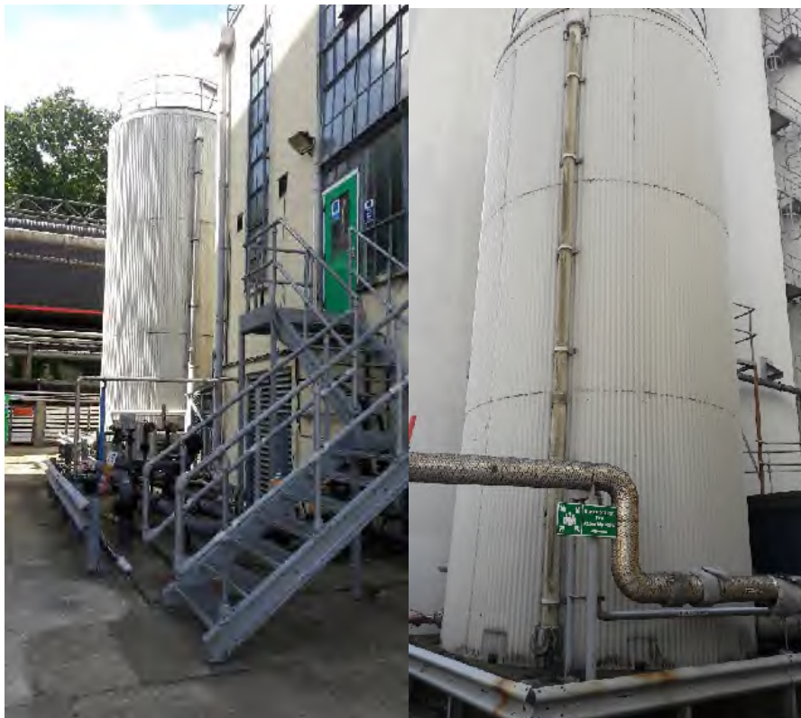
Plate 8: Reverse Osmosis water tank adjacent to the mustard seed silos
