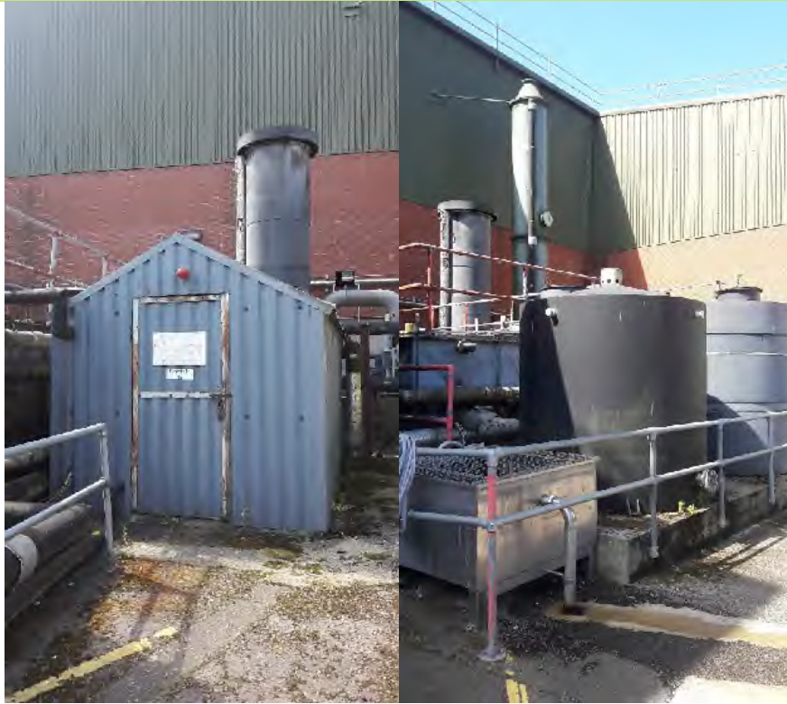
Plate 7: Borehole 'D' and associated air stripping / water treatment plant for the removal of PCE to the north of building 224
