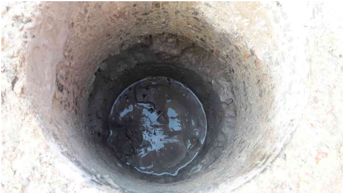
Plate 4: Very thick concrete at WS27, Area 10.
