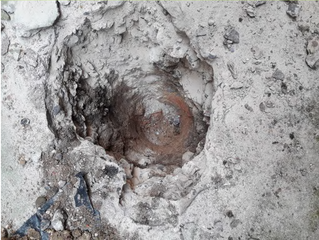
Plate 11: Concrete obstruction at 0.4m at HP1, Area 15.
