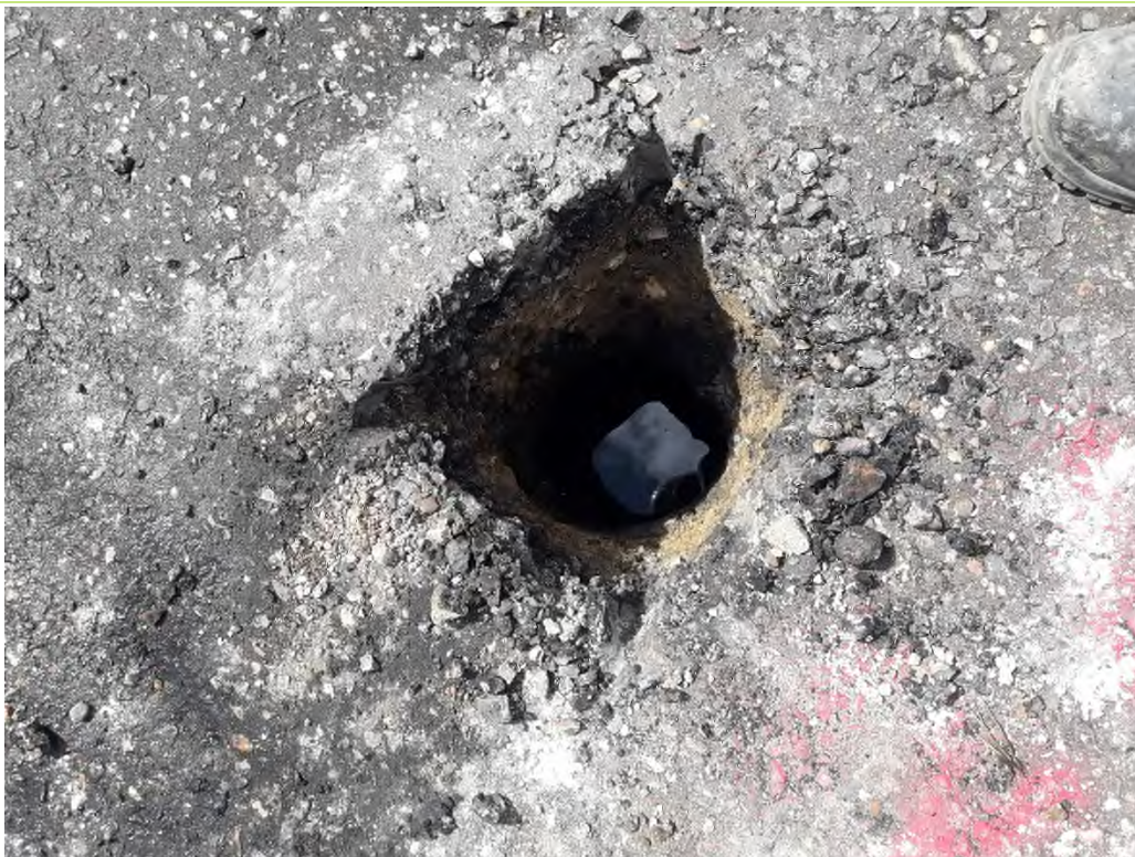
Plate 8: Very shallow groundwater below 0.8m at WS24, Area 10.
