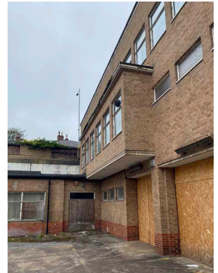
Figure 5.83 Main range of the station. Garage doors have been boarded up
