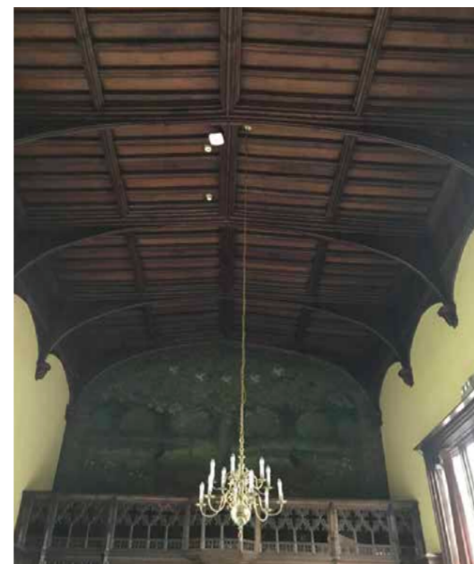
Figure 5.28 View of 19th century gallery and wall painting inserted during the 1880s restoration of the Guest Chamber
