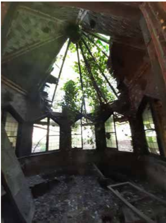
3.7 Rustic Summer House (non-designated) in extremely poor condition
