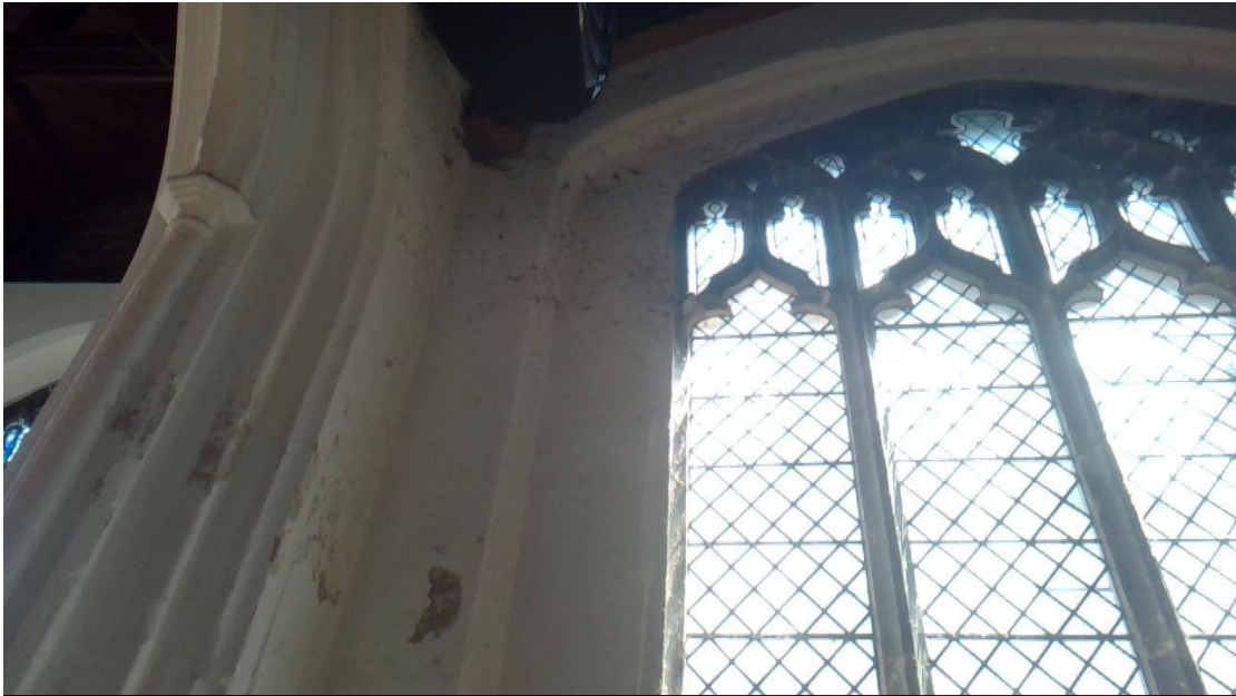
Cobwebs to walls
